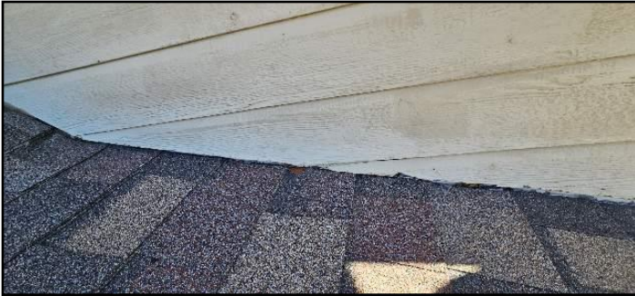
18. Siding not cut back
