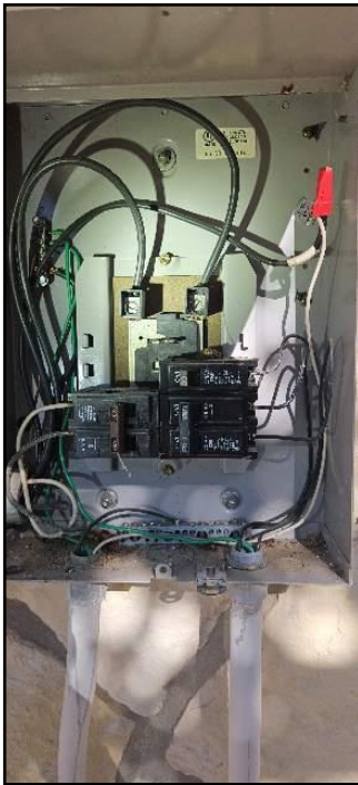
71. Non standard installation of the neutral wire
