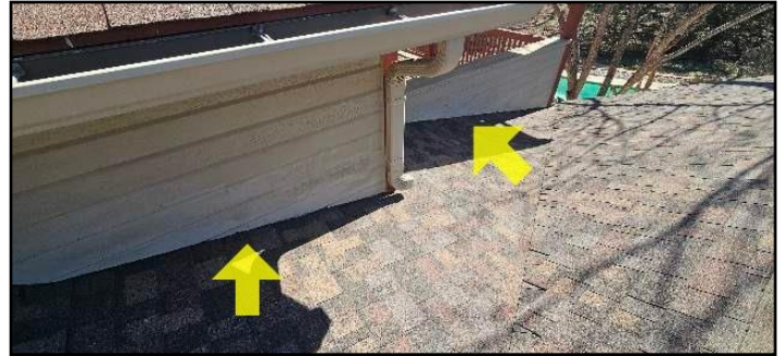
19. Siding not cut back
