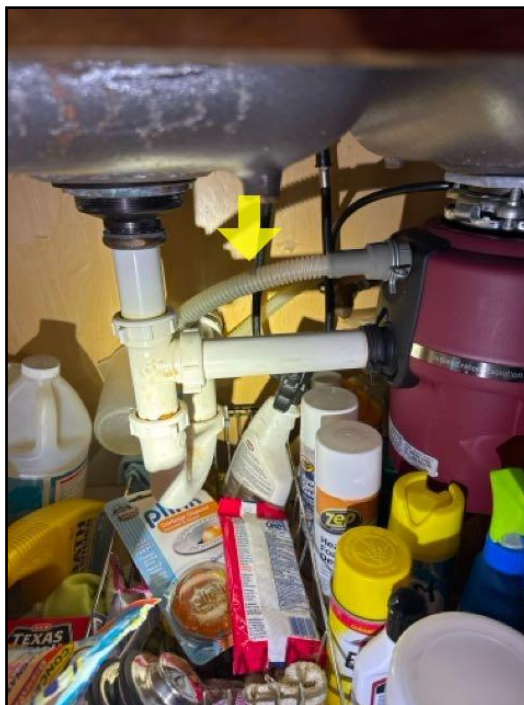
123. Backflow prevention high loop missing
