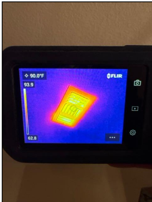
81. Heat pump operative
