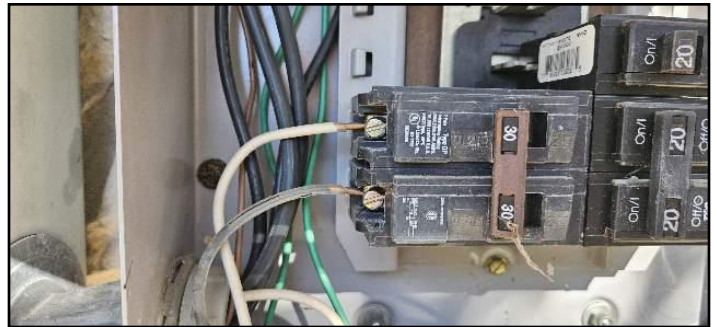
70. White wires connected to breakers not id
