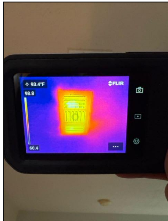
82. Heat pump operative
