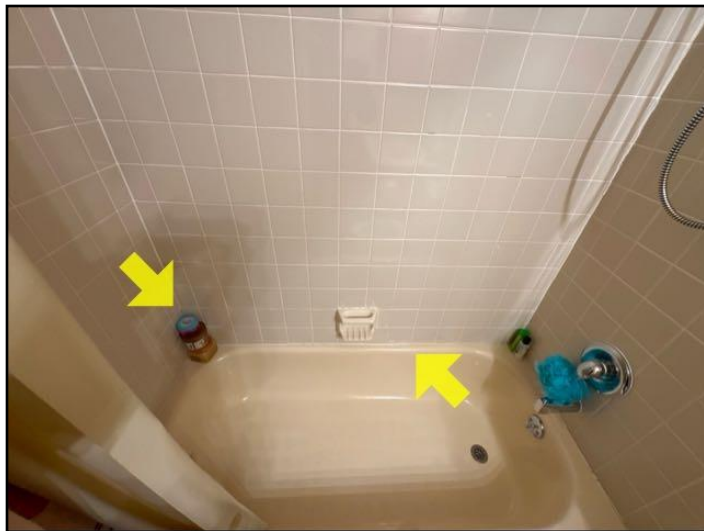
112. Grout loose, missing or deteriorated
