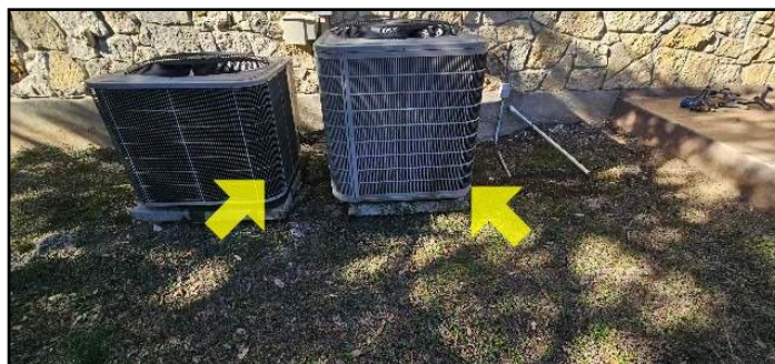
40. Improper slope or drainage
