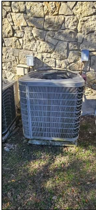
93. 2011 Air conditioner 4-ton unit
