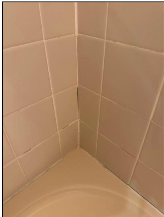
111. Grout loose, missing or deteriorated
