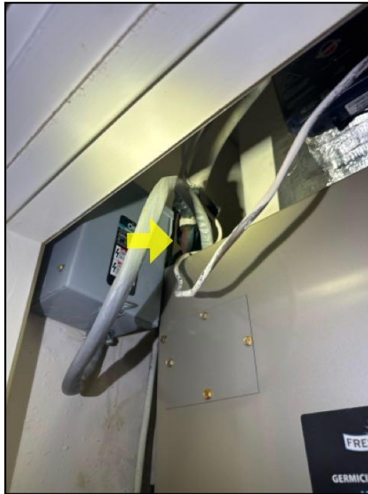
97. HVAC refrigerant Insulation deteriorated,...
