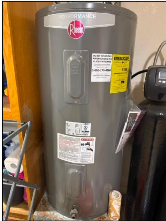
100. 2023 Rheem 50 gallon electric water heater
