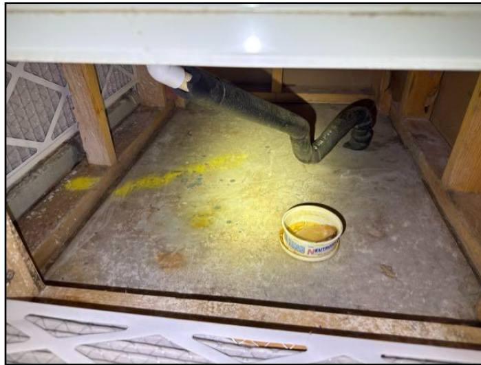
96. No drain/safety pan installed at the HVAC...
