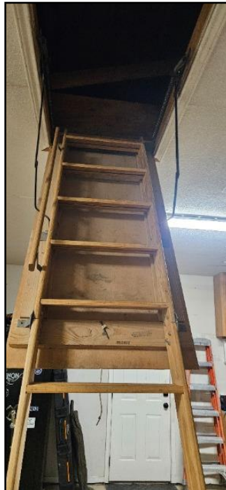
98. Plywood not fire rated
