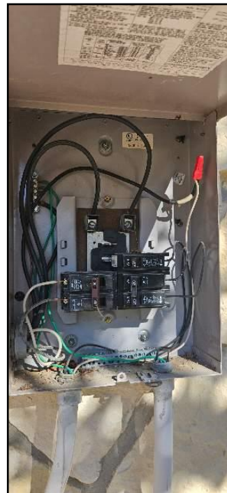
62. Breakers - exterior wall
