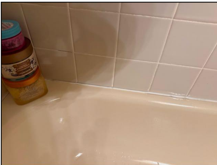
109. Grout loose, missing or deteriorated
