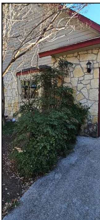
37. Trees or shrubs too close to building
