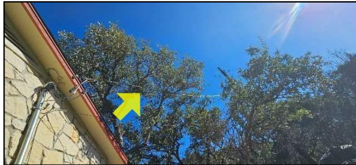
65. Branches / vines interfering with wires
