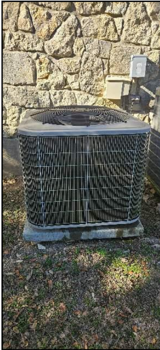
91. 2011 Bryant air conditioner 2-ton unit
