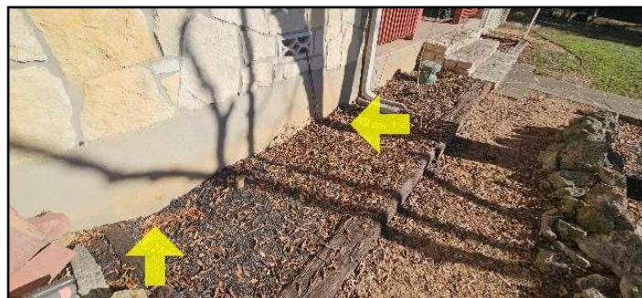
39. Improper slope or drainage
