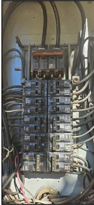
67. Box not bonded to ground
