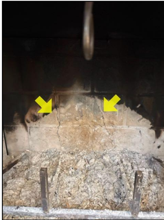
90. Cracked masonry or refractory
