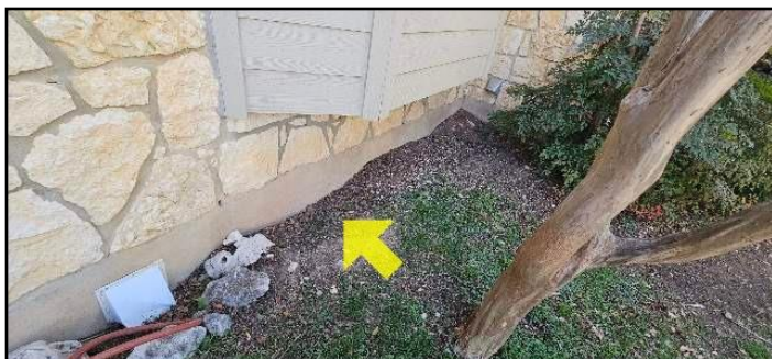
38. Improper slope or drainage
