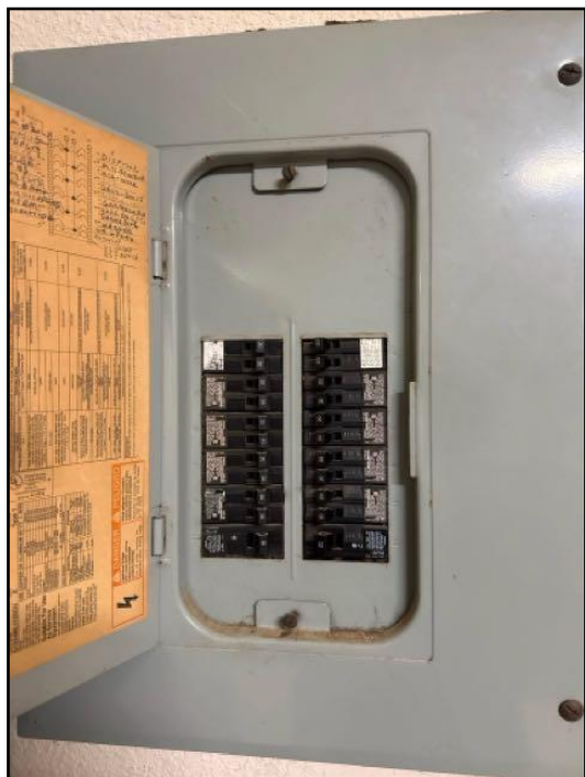
63. Auxiliary electrical panel
