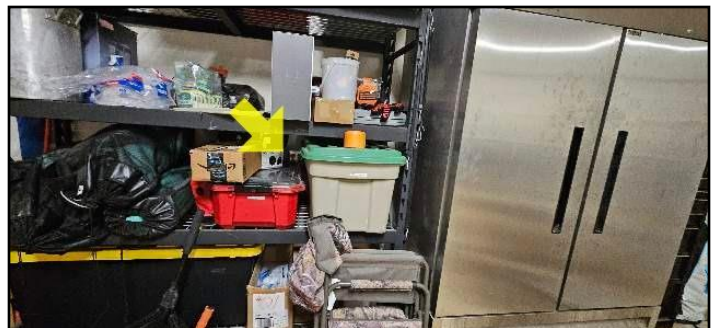
78. Garage GFCI missing
