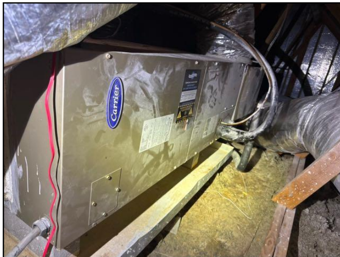
87. Heat pump operative
