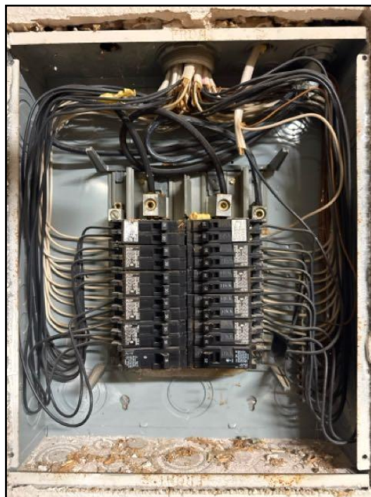
64. Auxiliary electrical panel
