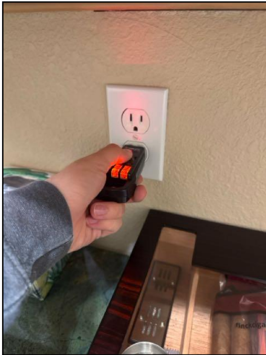
75. Bathroom GFCI missing
