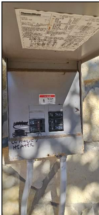
61. Breakers - exterior wall
