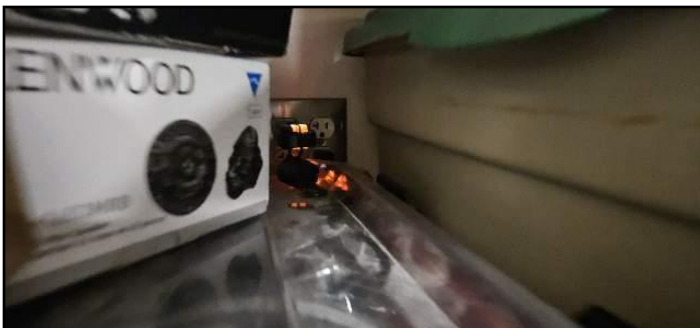
77. Garage GFCI missing
