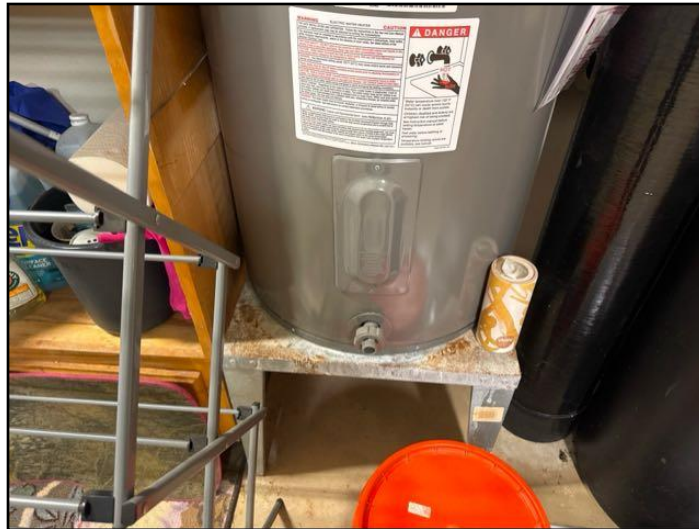
102. Safety pan and drain missing
