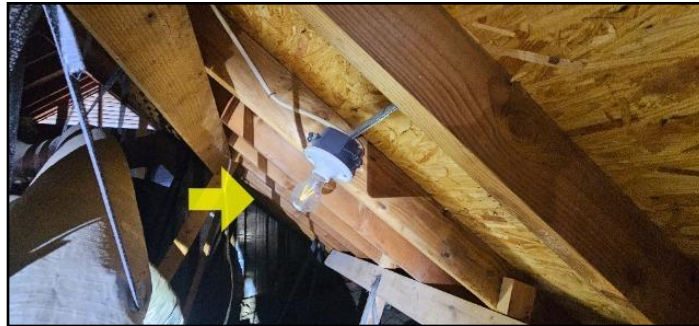
79. Exposed to mechanical damage (No cage or...
