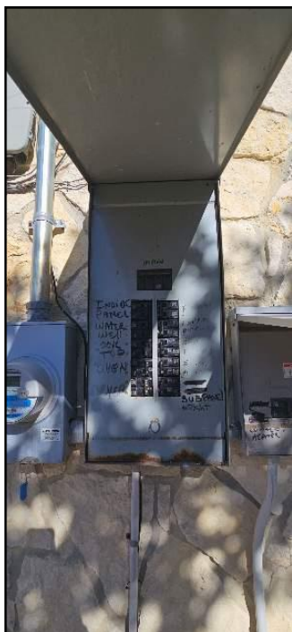
59. Main electrical panel
