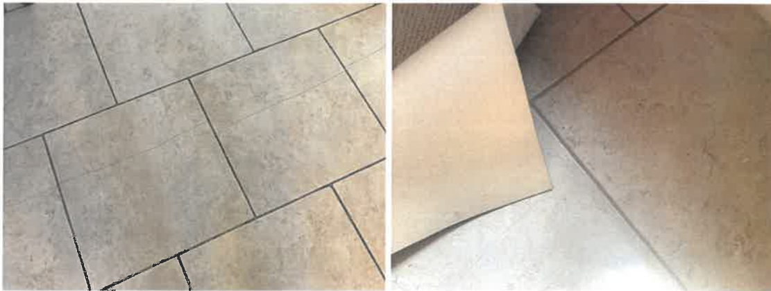
Pictures 1 and 2: Tile cracks.
