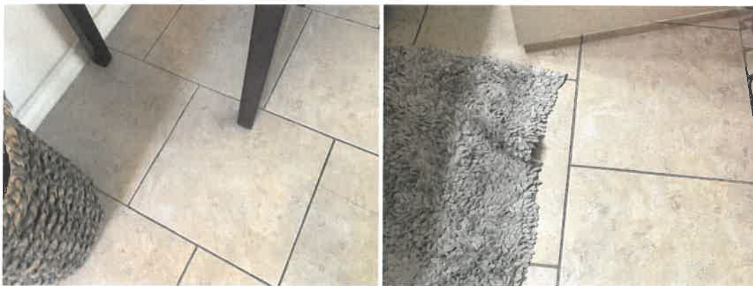
Pictures I1 and I2: Tile cracks.
