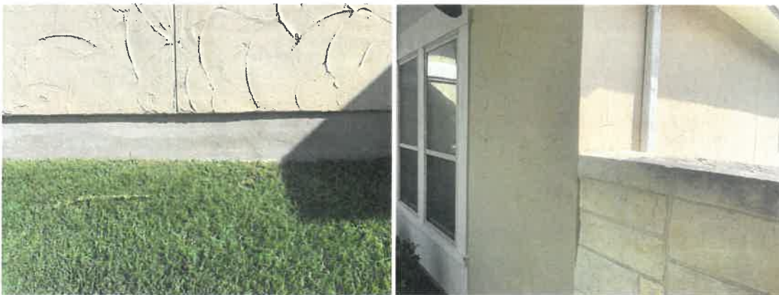
Pictures E1 and E2: Minor foundation curing crack. Front fence subsidence.
